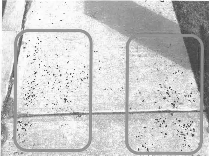
Photo 3 – Typical view of Medium Deterioration.
