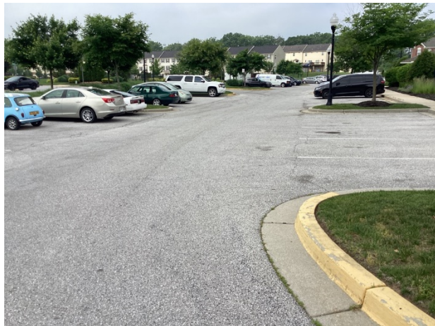
Clubhouse parking area overview Note: Previously sealed cracks.
