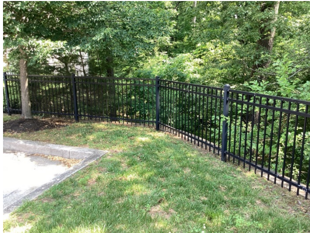
Aluminum railing overview Note: Finish deterioration.
