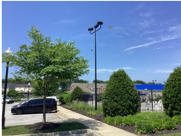
Light pole and fixtures
