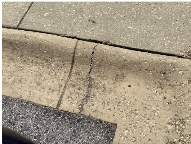
Curb and gutter cracks
