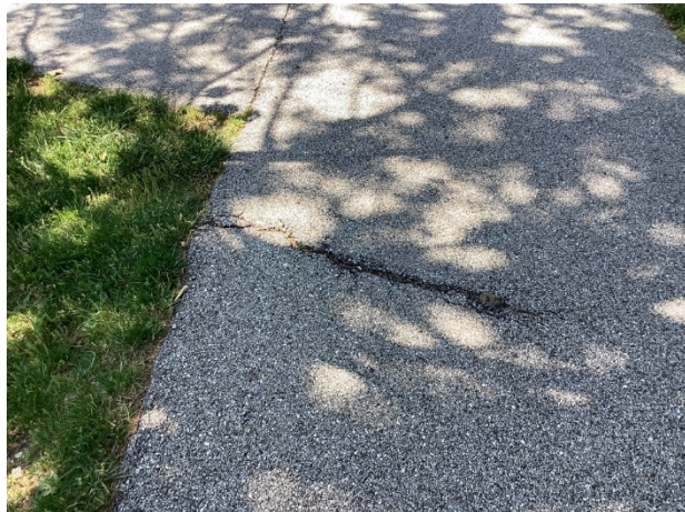
Walking path cracks and settlement
