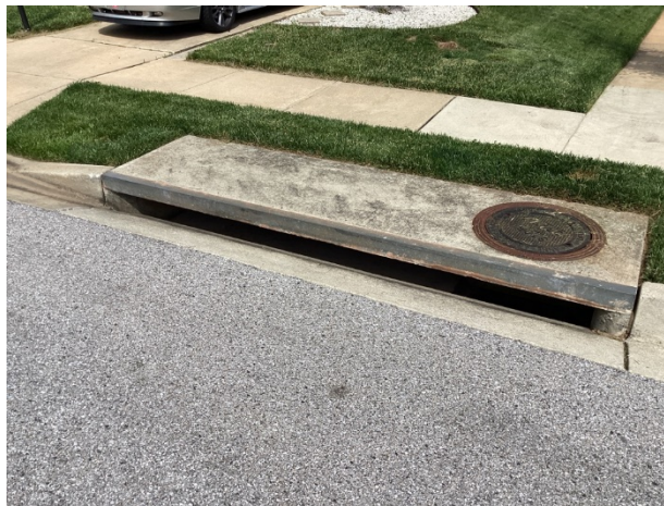
Typical townhome street and parking area catch basin
