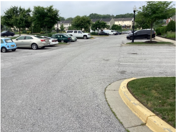
Clubhouse parking area overview Note: Cracks.
