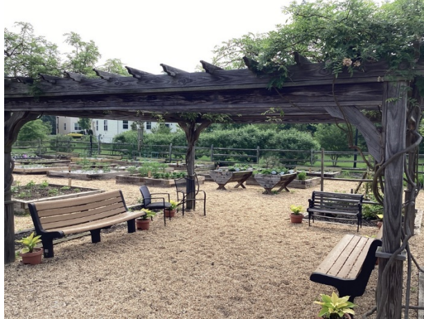
Wood pergola overview Note: Minor wood deterioration.
