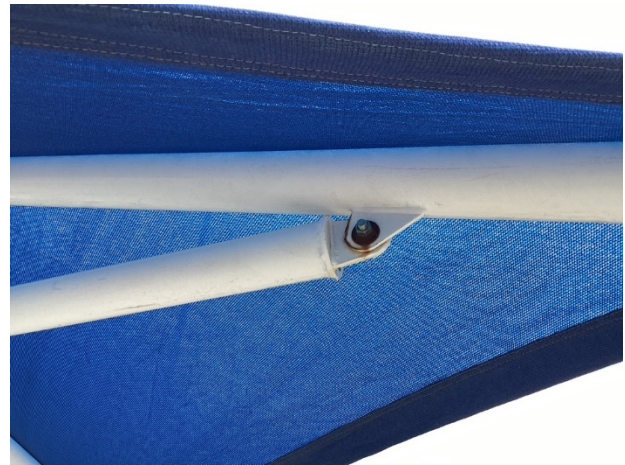
Fastener rust at connection
