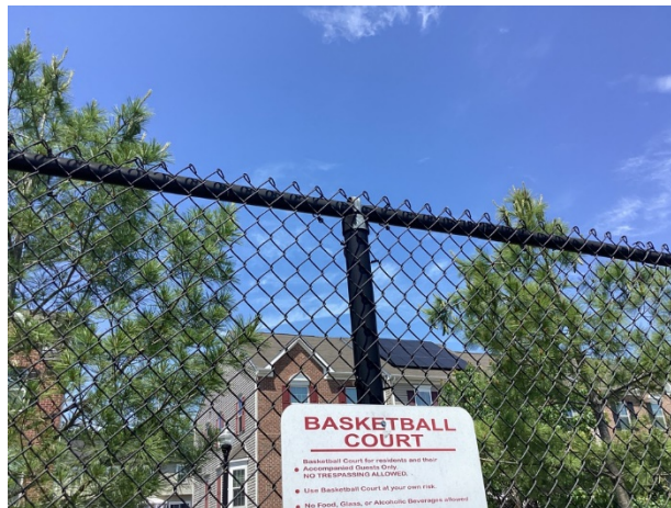
Finish deterioration at top of fence
