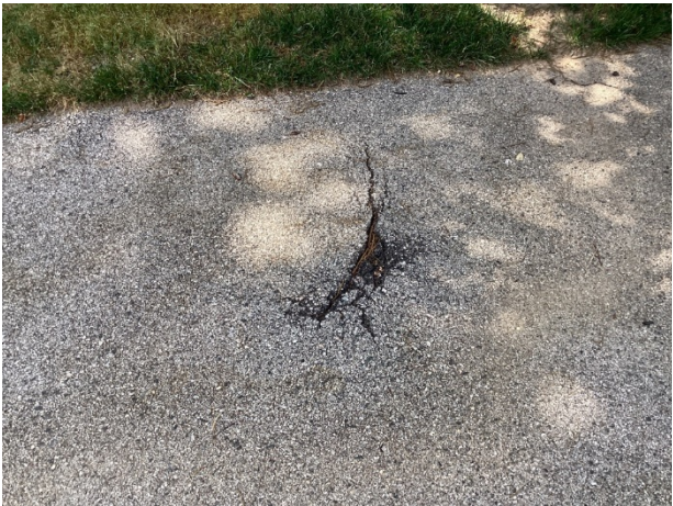
Walking path crack
