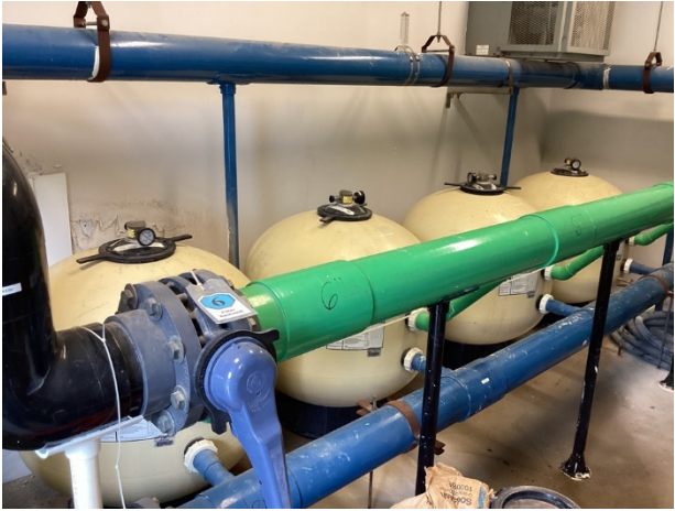
Pool filters and valves
