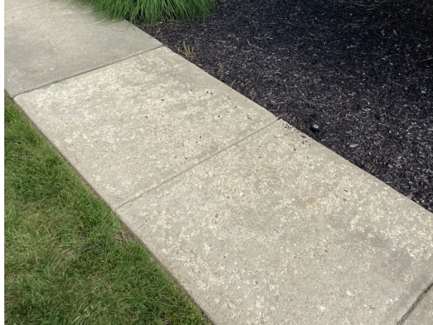
Scaling at Clubhouse sidewalk
