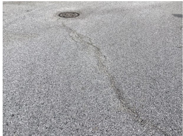
Section B and C pavement cracks
