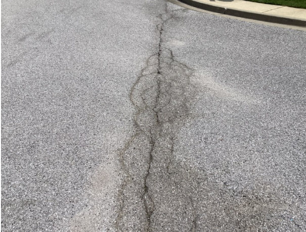
Section B and C pavement cracks
