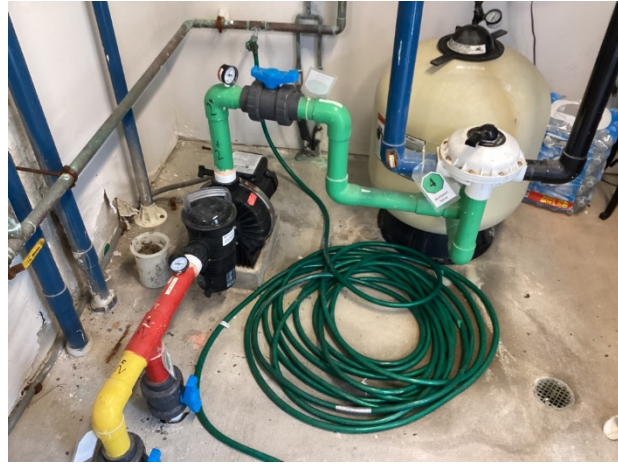
Pump and filter
