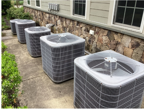
Split system condensing units
