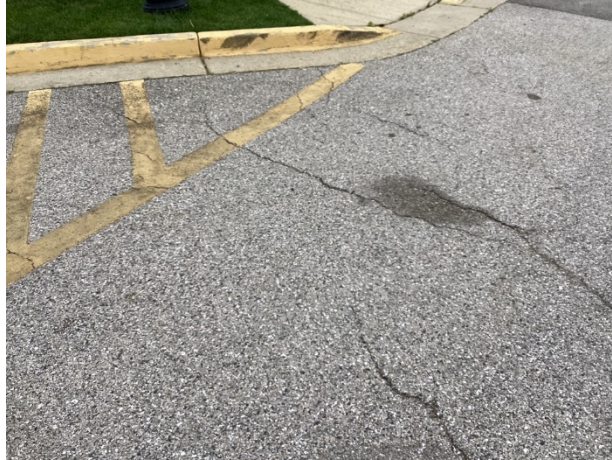
Clubhouse parking area cracks
