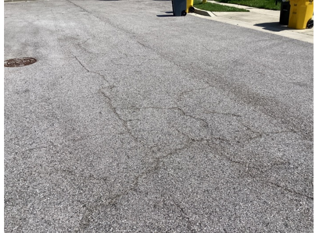
Section B and C pavement cracks
