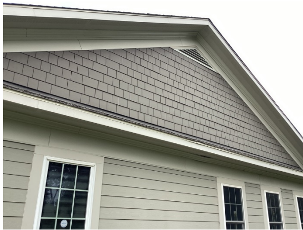
Fiber cement walls, trim, soffits and fascia
