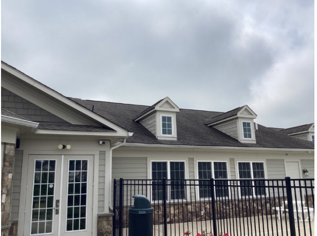
Clubhouse roof overview Note: Stains.
